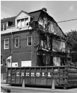
Burned homes torn down
